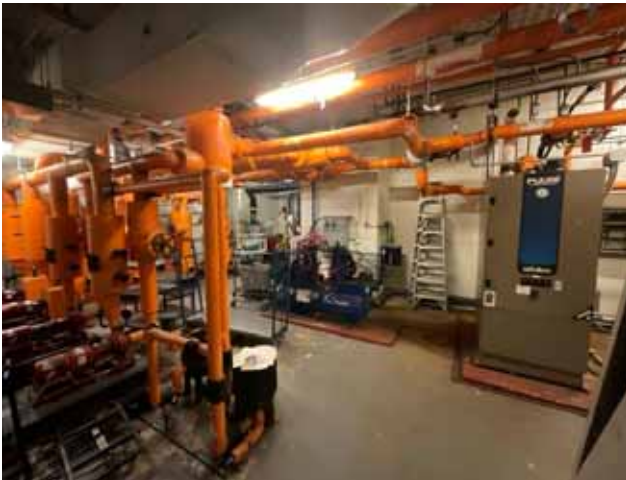
9 - BOILER ROOM OVERVIEW
