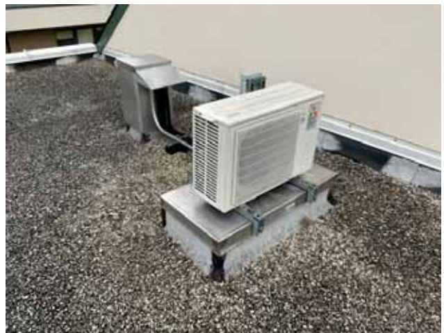
12 - SPLIT SYSTEM DUCTLESS
