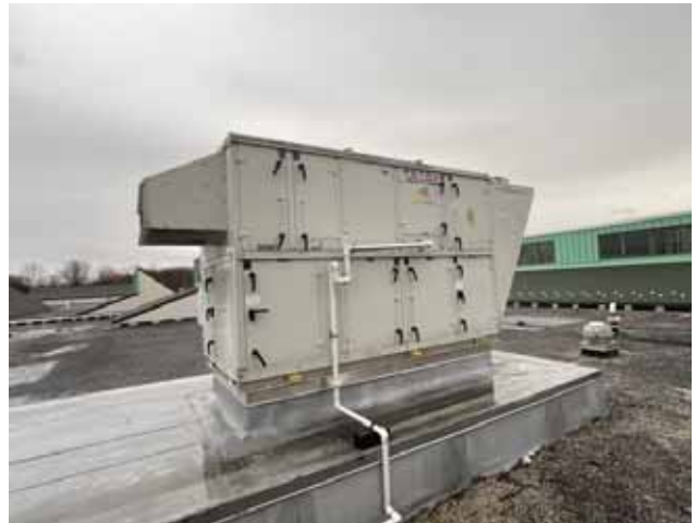
10 - ROOFTOP PACKAGED UNIT
