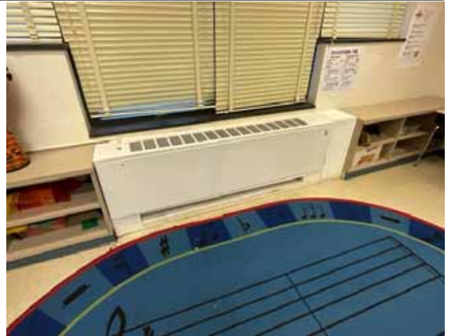
14 - CLASSROOM UNIT VENTILATOR
