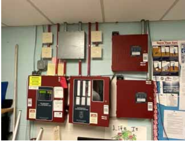
19 - FIRE ALARM PANEL
