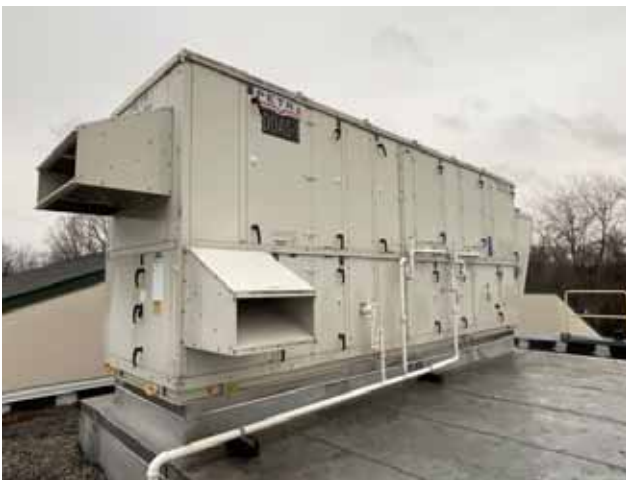
11 - ROOFTOP PACKAGED UNIT
