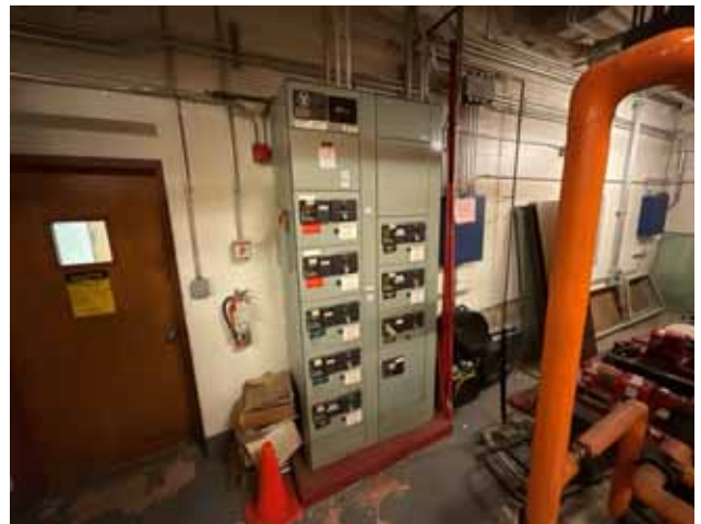
16 - MOTOR CONTROL CENTER
